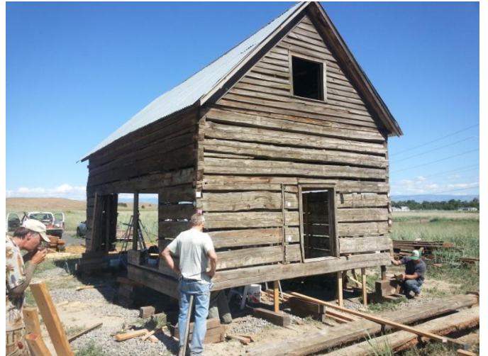
Top: Eric Sederburg making the critical dovetail corner cut in a replacement log, with help from Jehenn Poirot & volunteer Ross Osborn. Below, the cabin starts to take shape again as the lower walls are reinstalled with additional help from volunteer Steve Smart.
